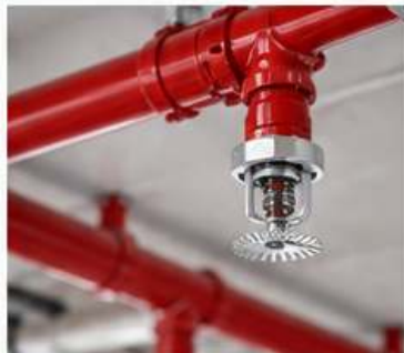
FIRE FIGHTING SYSTEMS
